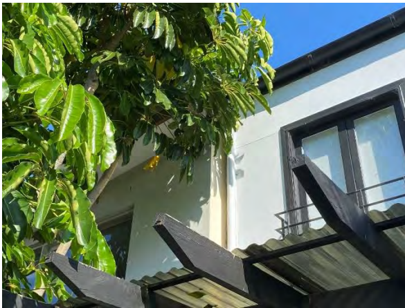
Figure 9: Interface of the existing rear elevation at the first floor with the terrace house at 56 Ruthven Street.
