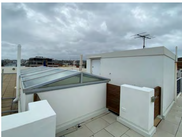
Figure 5: Southerly view of the roof terrace used by neighbouring units and accessed via different internal stairs.
