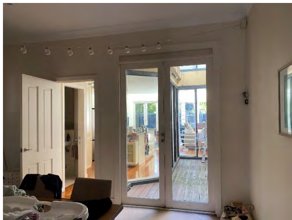
Figure 3: Existing void at the ground floor.
