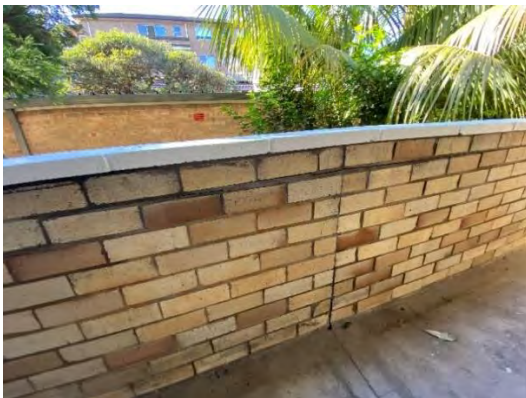
Figure 3: Cracks in the brickwork of existing balustrade.
