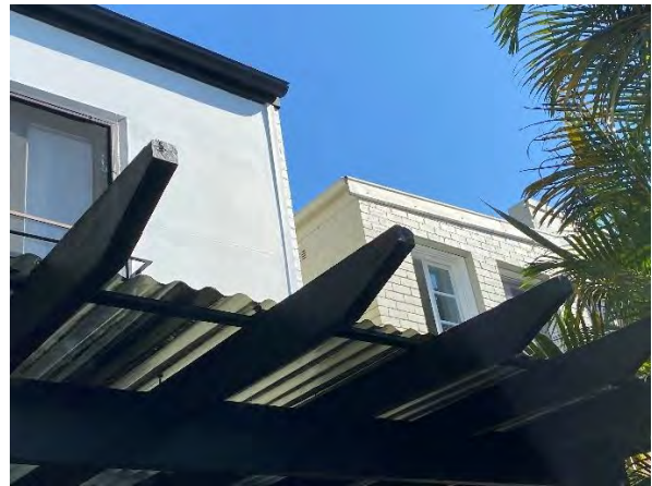
Figure 10: Partially detached interface of the existing rear elevation the first floor with the terrace house at 52 Ruthven Street.
