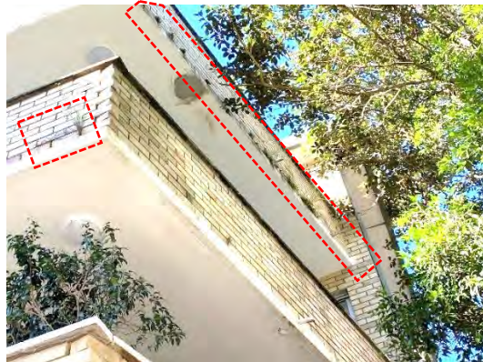
Figure 4: Weeds growing in the cracks in the brickwork.
