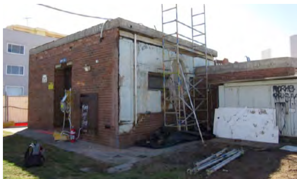
Figure 4.96: Arched window to the Sewage Pumping Station exposed during the 2015 works. Source: JRA
