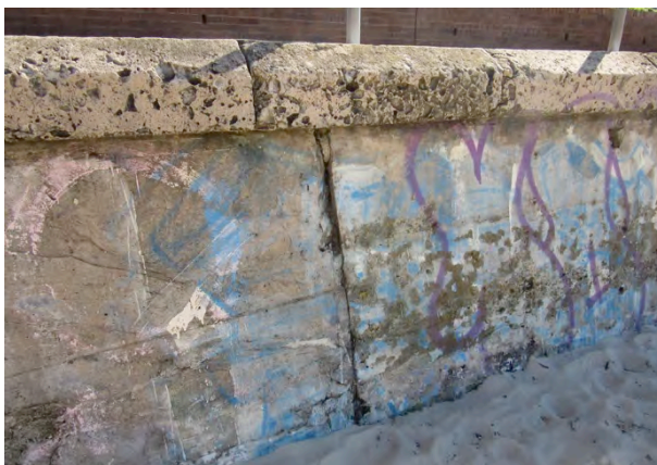
Figure 4.34: Sea wall showing construction joints in wall and coping which is in about 1m lengths. Source: JRA
