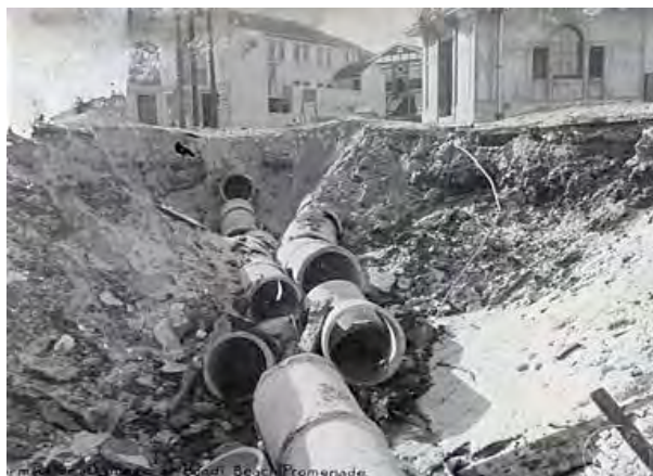
Figure 2.79: February 1929 View showing the low level pumping station (top right) and stormwater damage that occurred shortly after completion. Source: WIL 128
