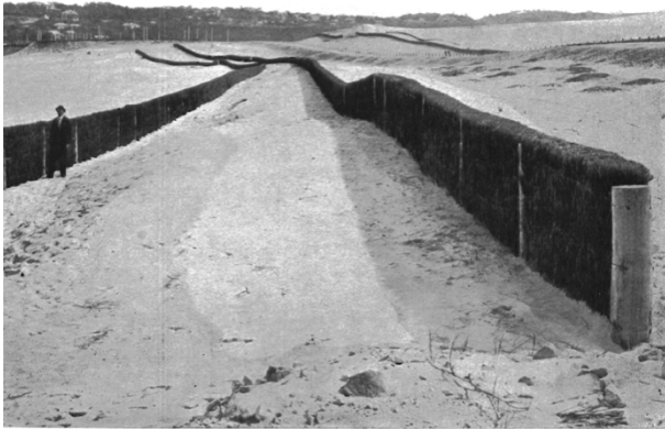
SHOWING GENERAL ARRANGEMENT OF FENCES PROTECTING THE ROAD.
