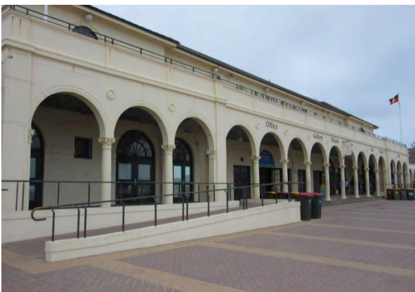
Figure 4.129: Close view of the pavilion arcade. The modern paving is raised. Disabled ramp on left. Source: JRA 2020
