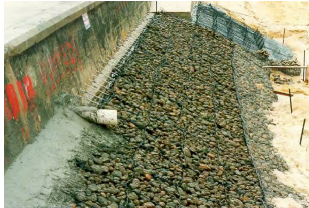
Figure 2.131: 1990 photo of revetment works in progress. Source: From paper by Lex Nielsen http://www.coastalconference.com/2012/papers2012/Lex%20Nielsen%20Full%20Paper.pdf
