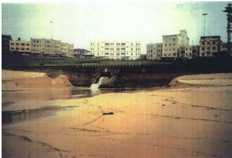
Figure 2.10 Old stormwater outfall, showing beach scour following storm event August 1986 (source PWD 1988)
