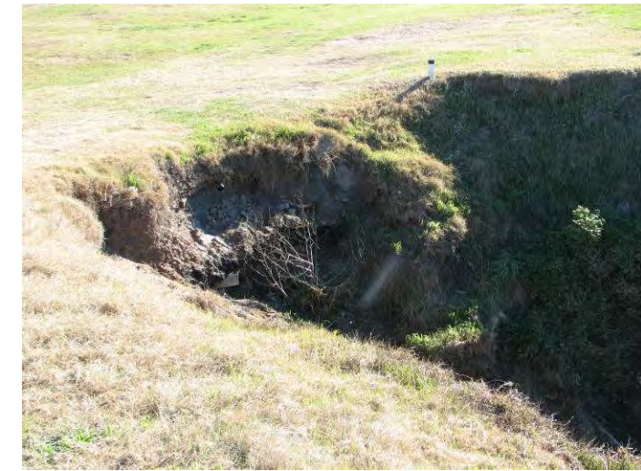
Instability of soil slope
