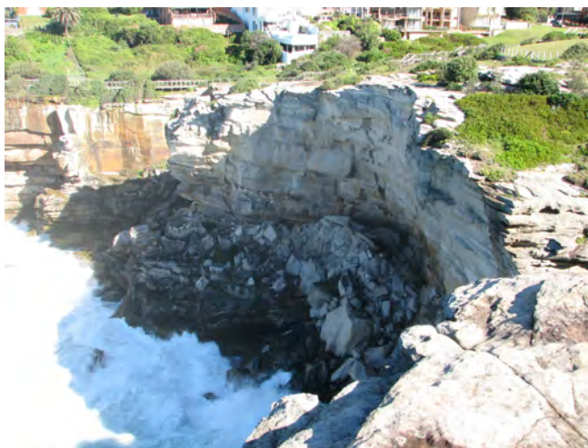
Figure 5.4 Collapse of cliff face overhang at Diamond Bay
