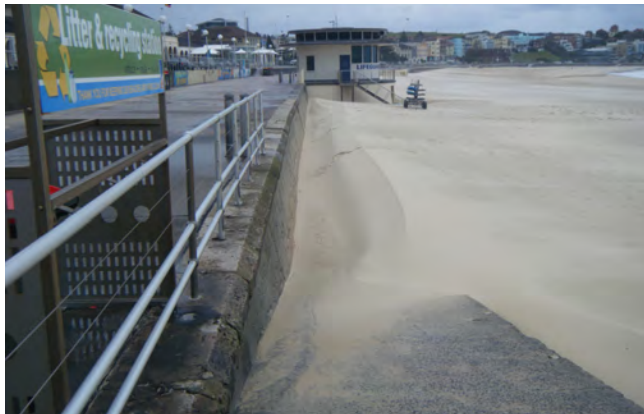
Figure 3.10 Scour in front of Bondi Seawall caused by stormwater runoff
