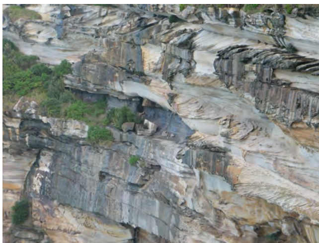
Figure 5.2 Cliff face failure onto cliff bench
