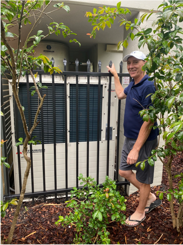
Strata Committee member and project manager David Walton with the Mitsubishi Q-Ton air-to-water heat pump
