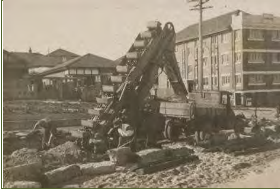
Figure 2.17: 'Barber Greene' excavator in operation on Campbell Parade, North Bondi. This undated image gives an idea of the types and depths of disturbance of the uppermost sandy soil profiles that are currently sealed below the current alignment of Campbell Parade (Waverley Image Library)
