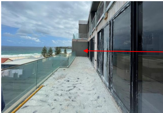
Figure 3: Existing Level 4 balcony showing the location of the relocated eastern external wall approved under DA-373/2023. See figures 5 & 6 for the approved and proposed section details.
